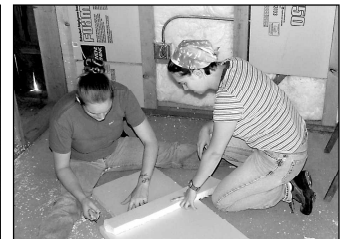
Volunteers Kathy VanWormer and Amy Folz cutting rigid insulation for interior wall.
